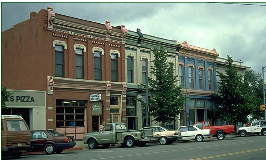
After rehabilitation, the row of buildings shown in the photograph above conveys a stronger sense of its historic character. Note that some old uses were retained, while other new uses were also introduced. Some incompatible alterations were removed and storefronts were appropriately reconstructed. (Fort Collins, CO)
