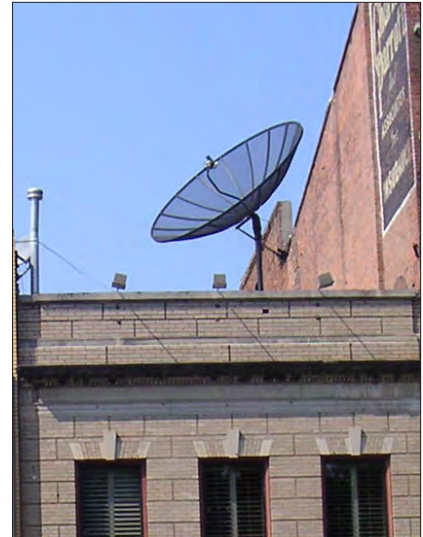
Minimize the visual impact of roof-top equipment on the public way. (Athens, GA)
