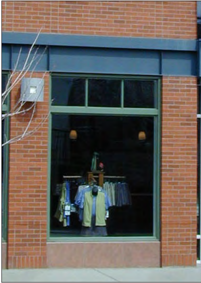
Contemporary building materials should be used in a manner that conveys a sense of scale similar to that seen in historic materials.
